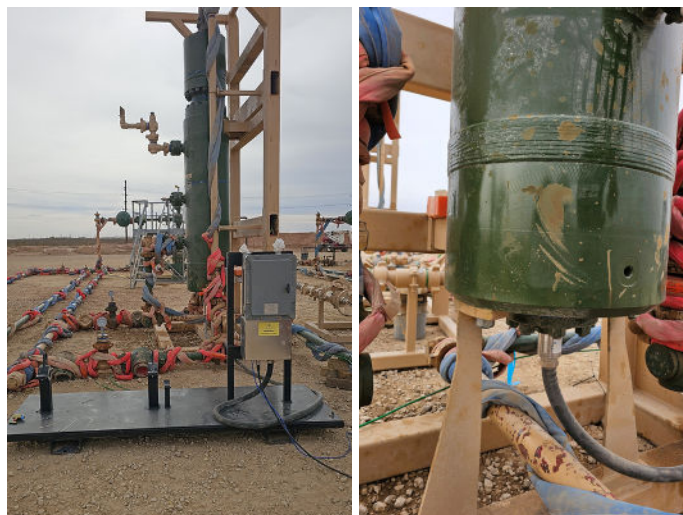
Picture 1 : ROCsole SoliDetect1.0 installation in ENERCORP Sahara Sand Cyclone.
